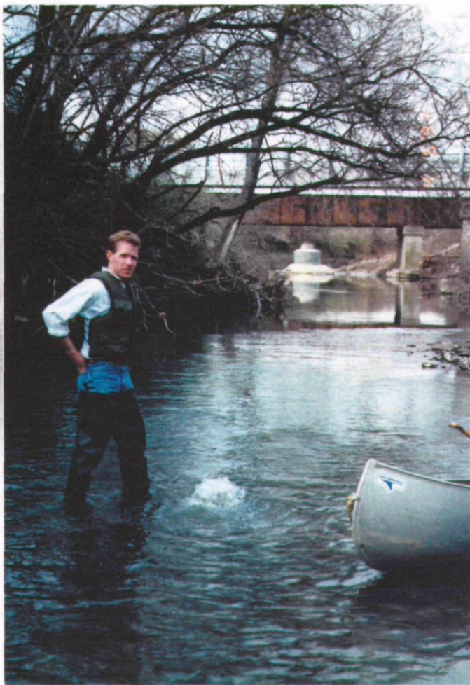
Plate 3. Sewer manhole located in the stream bed of Mill Creek discharging sewage into the stream downstream of the G.E. tributary.
